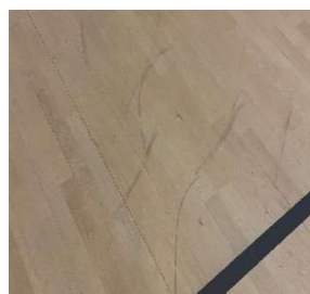
Damaged caused by marking shoes used on court.
